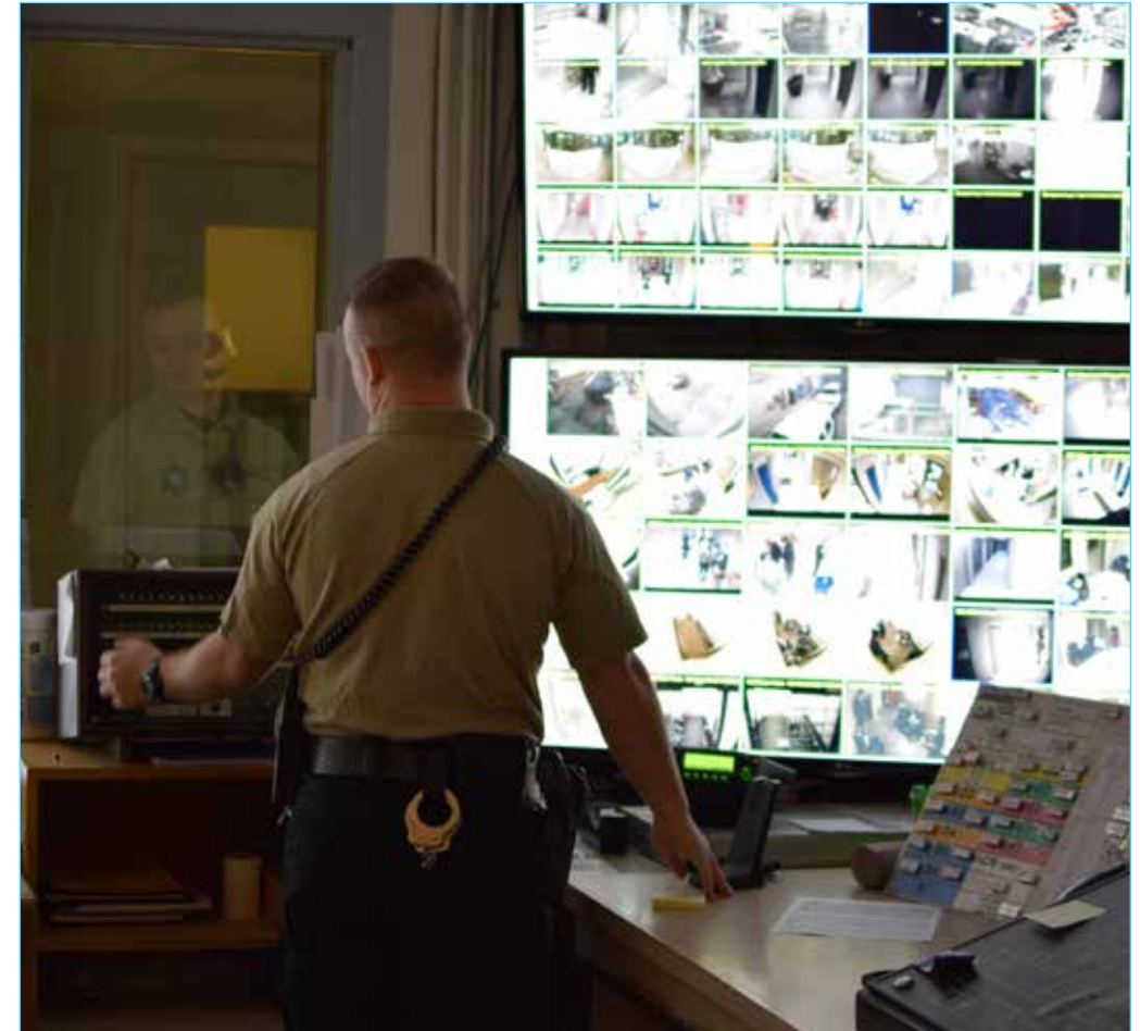
Escambia County Main Jail Central Control
