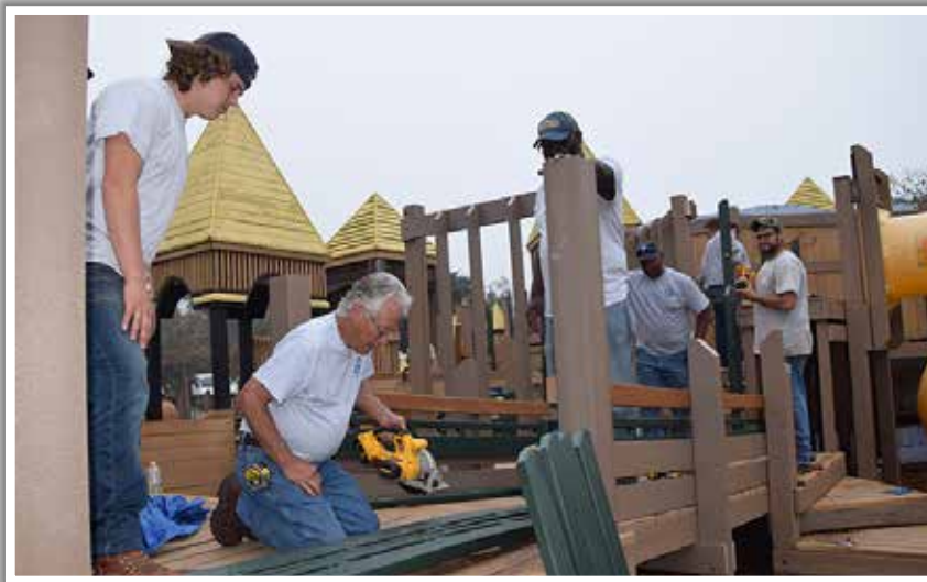
Above: Volunteers were a vital part of the Perdido Kids Park renovations.
